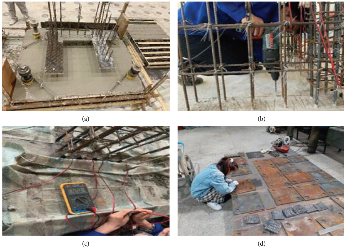
FIGURE 9: Template support for preliminary work. (a) Pre-embedded thread sleeve. (b) Chiseling the connection surface. (c) Detection strain gauge. (d) Making embedded parts.
