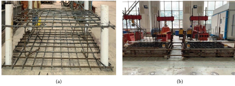
FIGURE 8: Manufacturing process of the base skeleton. (a) Base reinforcement skeleton. (b) Bottom supporting mold.
