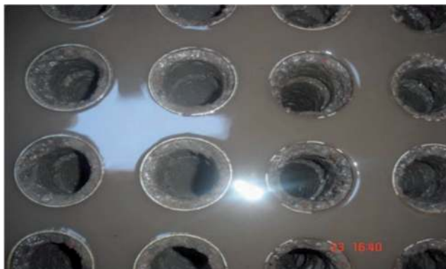
Figure 3. Soot deposits inside APH tubes.
