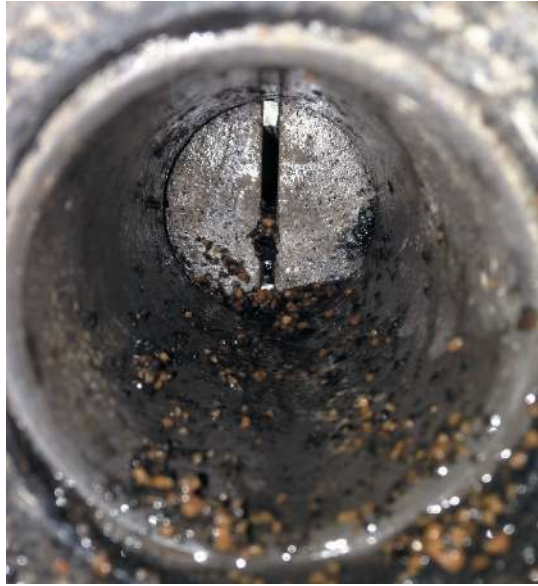
Fig. 15. Fracture opening (3 mm) partially plugged
