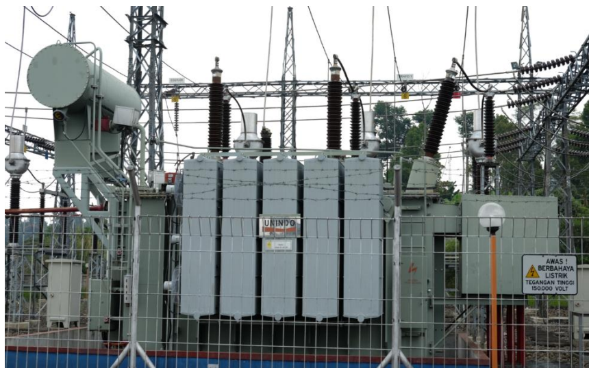
Figure 1. Example of 150 kV transformer used in this study
