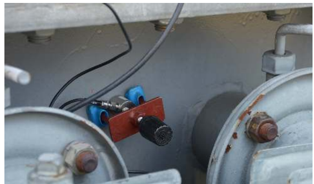
Fig. 4. AE sensor attached to the transformer – general view.
