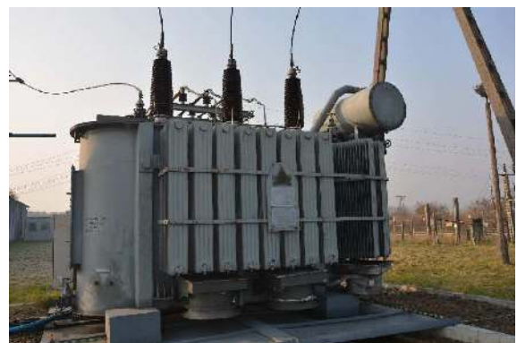
Fig. 10. Electrical power transformer 115/16.5 kV used for research – general view.
