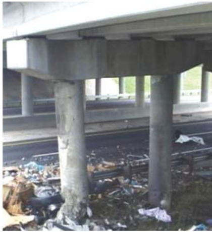
FIGURE 11: Failure mode of the pier of [2].
