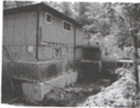
Figure 3: A strip foundation was performed under an existing wall in a steel frame structure by part by part method
