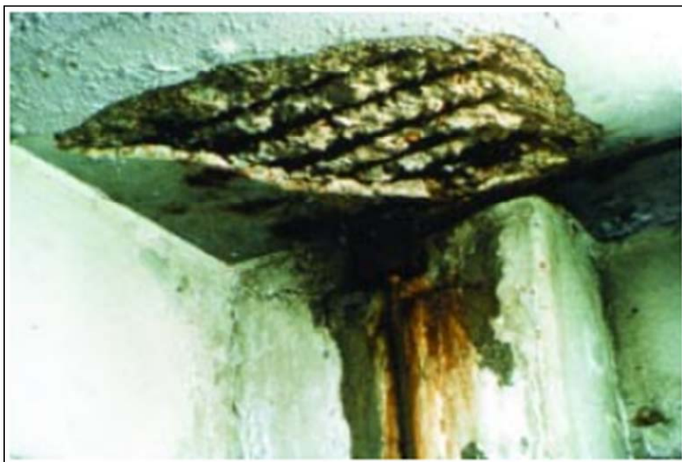
Figure 1. Corrosion of reinforcing steel is the most common cause of concrete deterioration [1].
