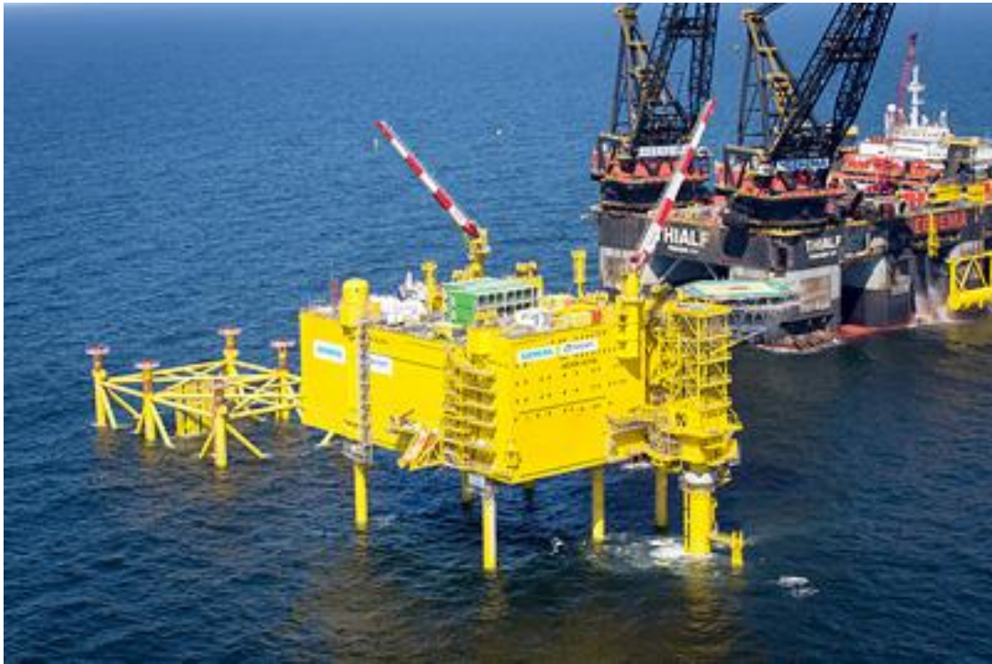
figure 5. The HelWin 2 foundation next to the HelWin 1 platform. (Used with permission of Siemens, www.siemens.com/press .)
