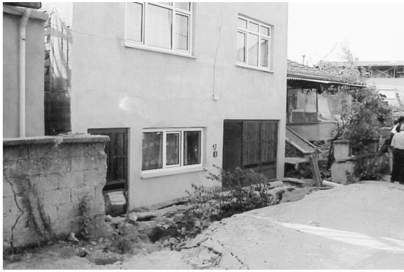
Fig. 8. Four-story building at Site F that underwent significant vertical and lateral displacement. Note gap between street and building that a felled tree was thrown in after the earthquake.
