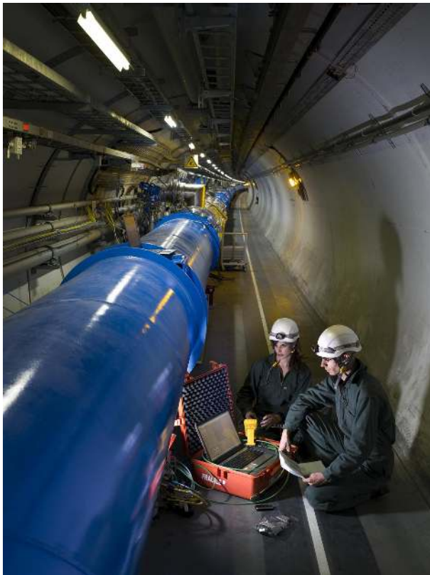
Fig. 26. LHC magnets in the LHC tunnel during electrical checks: in blue are the main dipoles, while the U-shaped tube visible in the middle connects a quadrupole to the cryogenic line.
