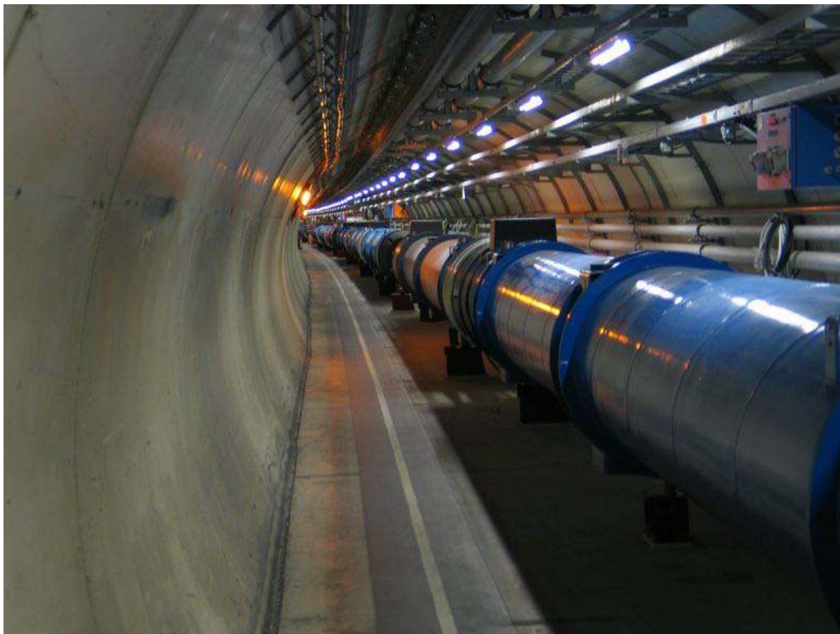
Figure 1. The superconducting magnets in the LHC tunnel
