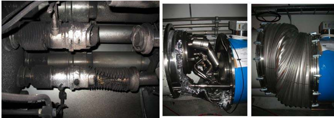
Figure 17. Pictures of the damaged zone after the incident. Left: close-up the interconnection where the first arc occurred, with vaporized cryogenic and vacuum pipes and soot deposited everywhere. Right: an interconnection between dipole (blue) and quadrupole (white) with interconnection bellow heavily deformed by displacement of the quadrupole against the dipole. Centre: the same interconnection after removal of the bellows.
