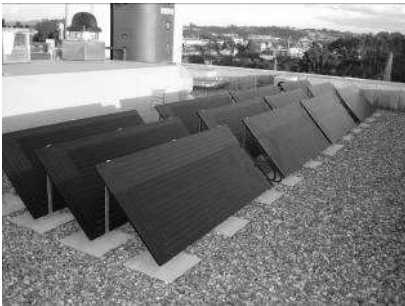
Figure 3. Hot water solar collectors (thermodynamic system).
