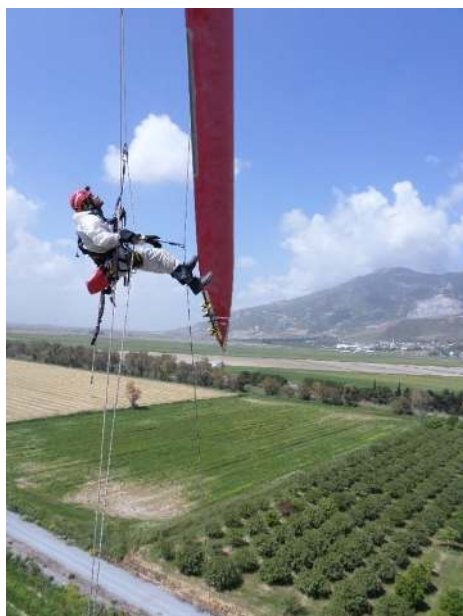
Figure 3. On-site repair of wind turbine blade. Reprinted with kind permission from Mira Rope Access, http://www.mira-ra.com , (accessed on 13 January 2021).
