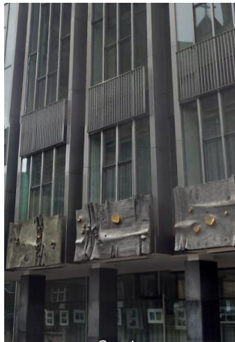
Fig. 8. The façade of the building with a large amount of highly reflective surfaces.
