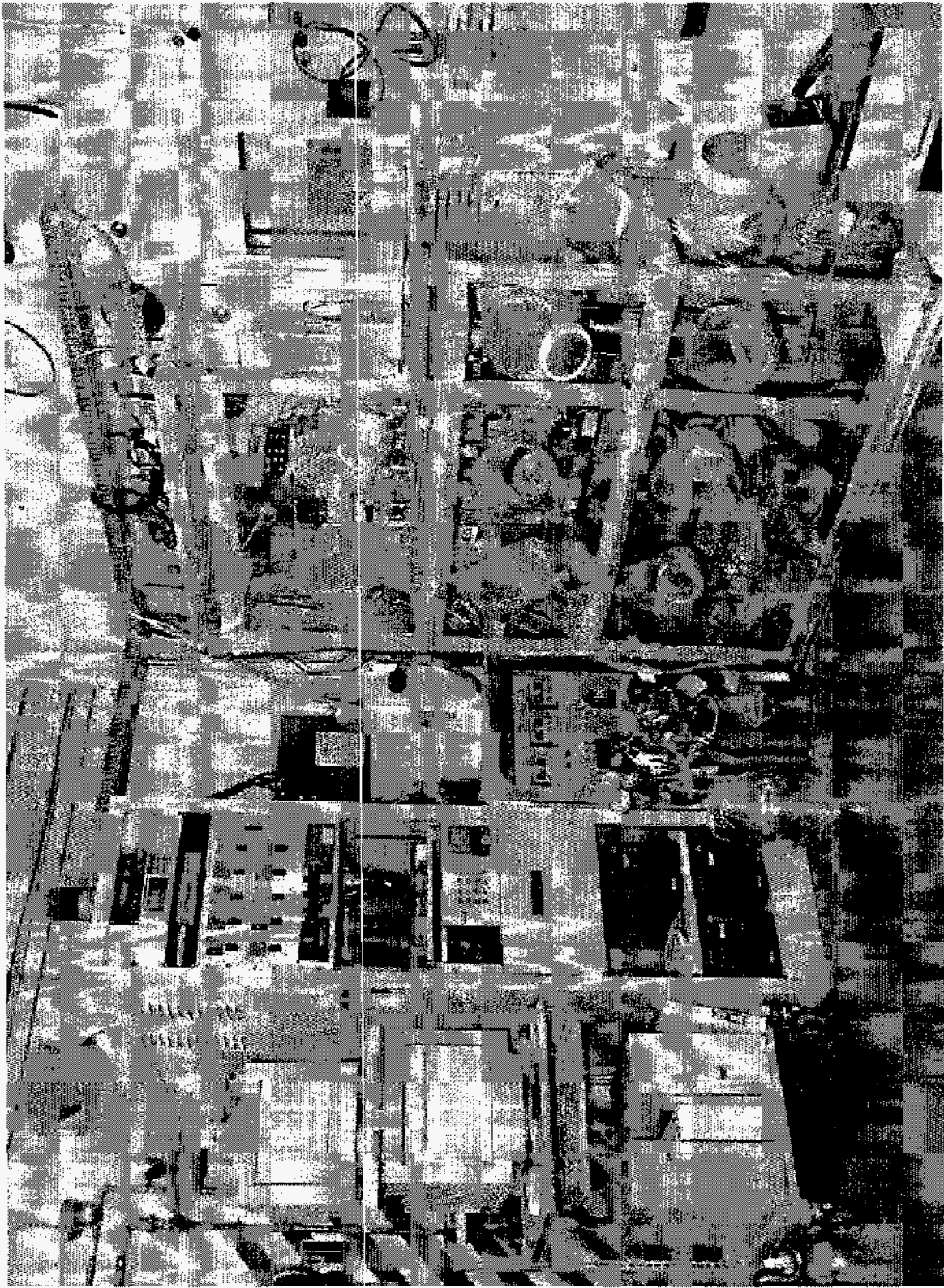
Figure 4. Photograph of Furnace System Equipment Outside G-Cell
