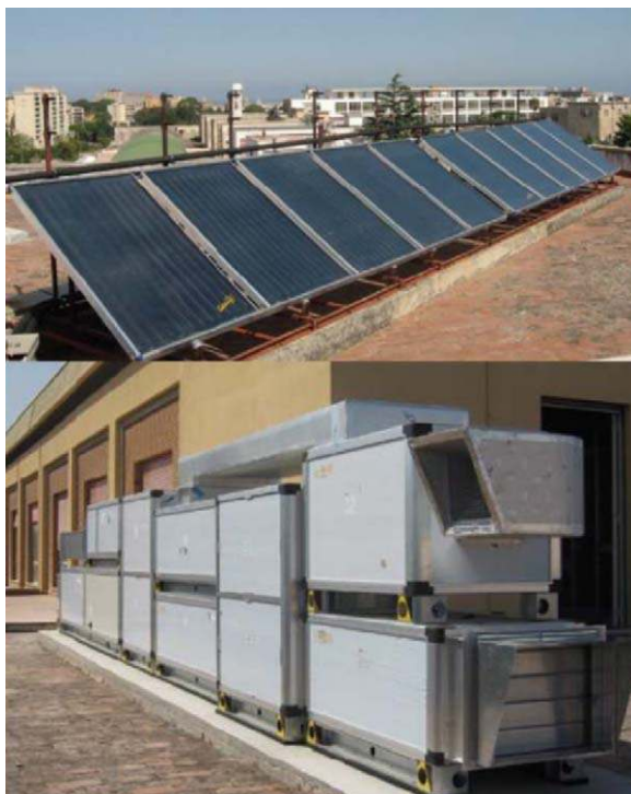
Fig. 19. Solar desiccant cooling system installed at University of Palermo, Italy [114].
