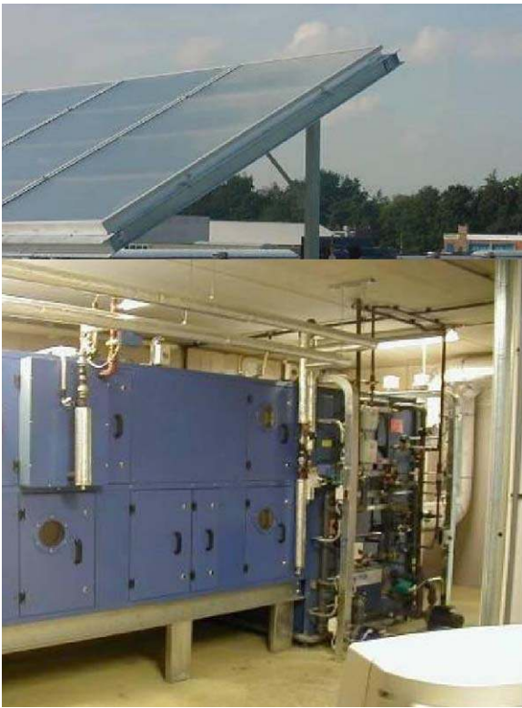
Fig. 25. Solar desiccant cooling system installed in Waalwijk, Netherlands [119].
