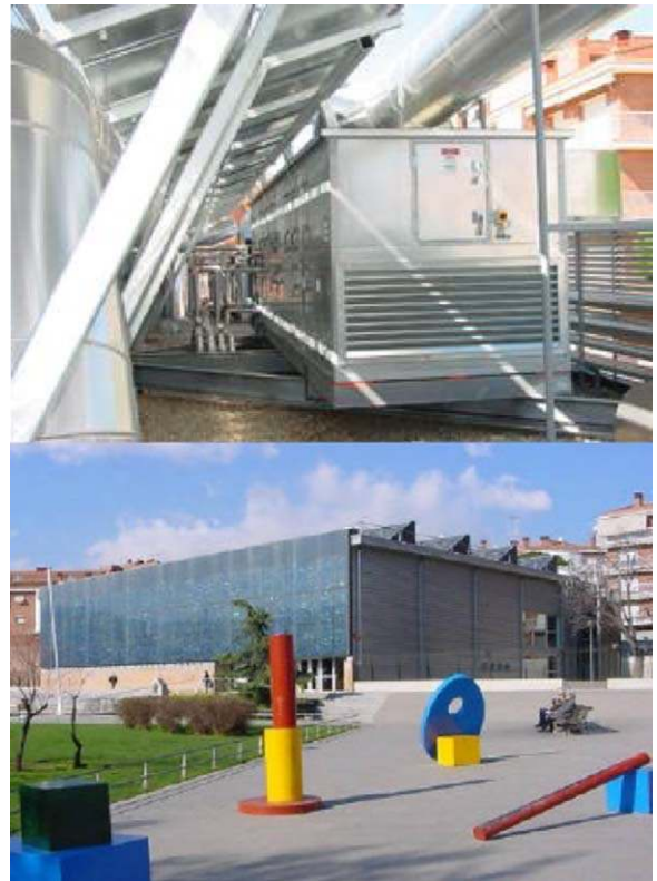
Fig. 23. Solar desiccant cooling system installed in Mataro, Spain [117].
