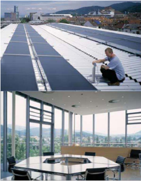
Fig. 21. Solar desiccant cooling system installed in Freiburg, Germany [117].
