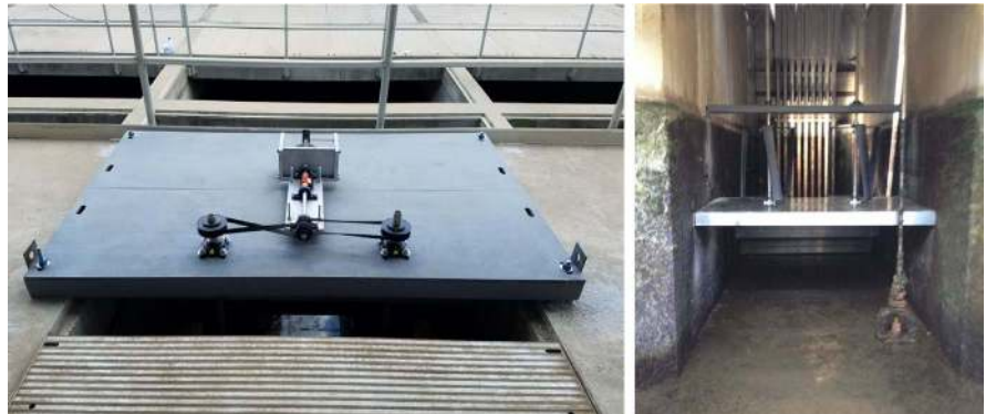
Figure 8. LHS, photograph of upper bridge as installed in RM Clayton including PTO and belt drive. RHS, photograph of downstream view of constriction, rotors and middle bridge.
