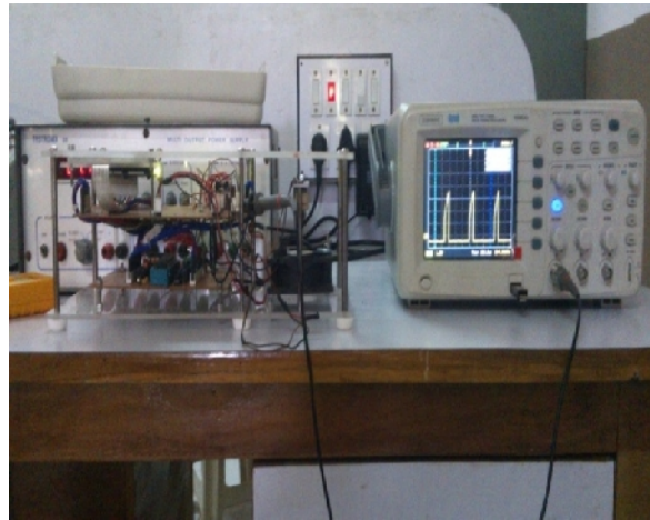
Fig 7: Overall view of system
