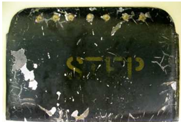
Figure 8. Chinook Fuselage Step Door is shown with flaked, chipped and cracked paint. It is approximately 20 cm by 14 cm
