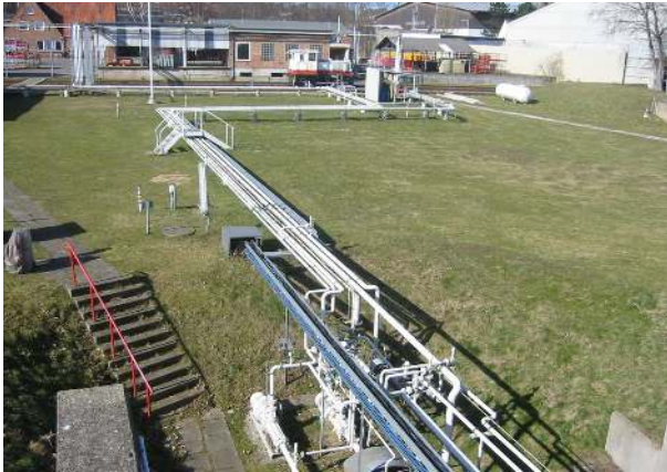
Figure 1. Pipelines of the company Boie GmbH in Lübeck
