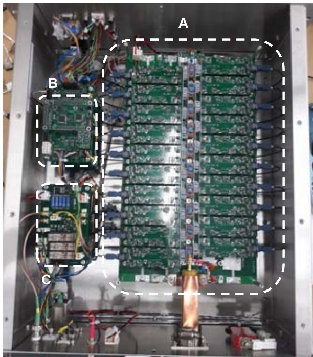
Fig. 7. Top view picture of the 19-inch rack of the generator. A: Marx generator, B: control \mu C board, and C: auxiliary power supplies and safety interlocks.
