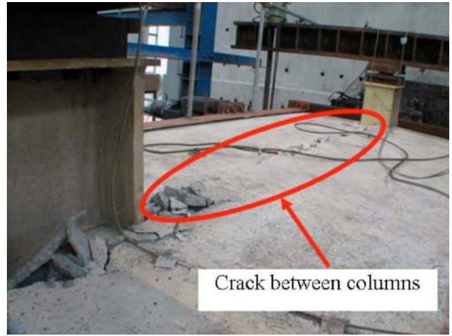
Fig. 12. Crack at top slab
