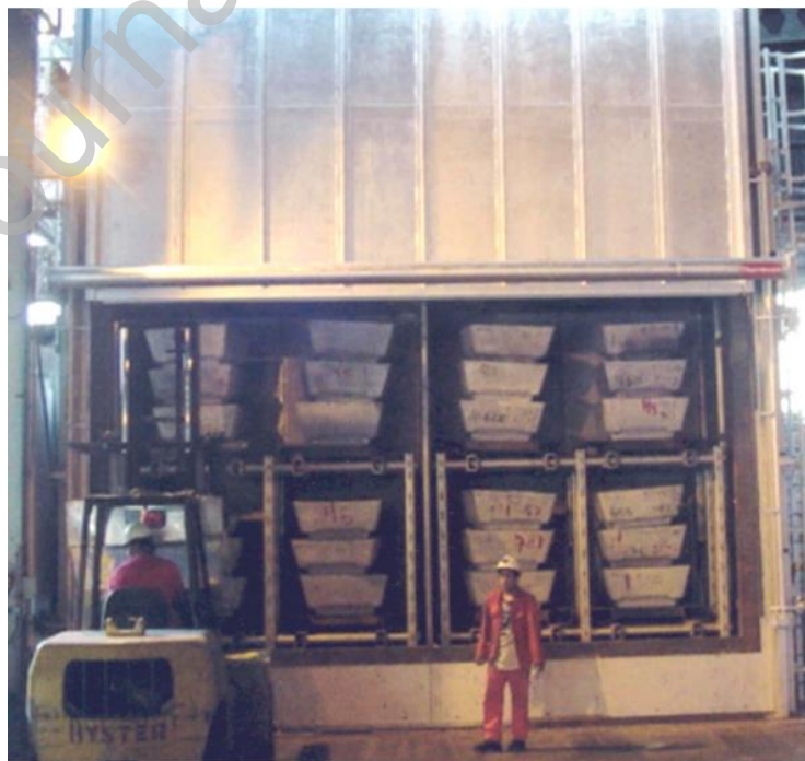
Figure 55: A chamber preheating aluminium scows using waste heat, reproduced from [243].
