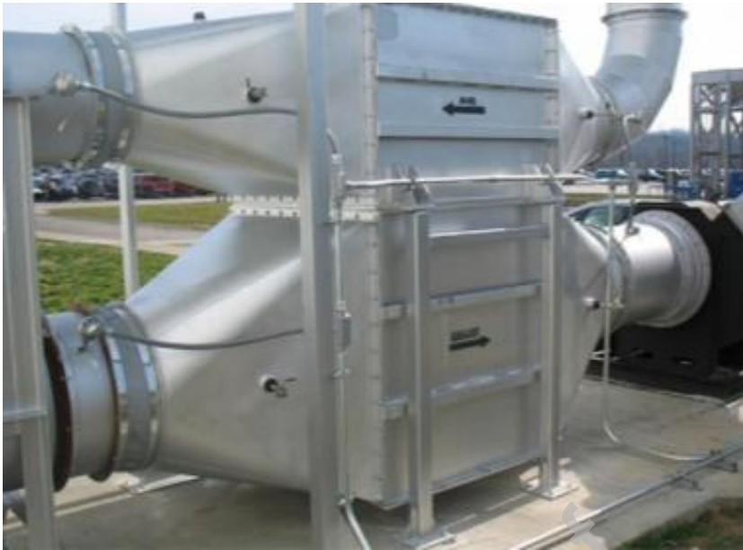
Figure 44: Heat pipe heat exchanger used to preheat combustion air. Taken from [213].
