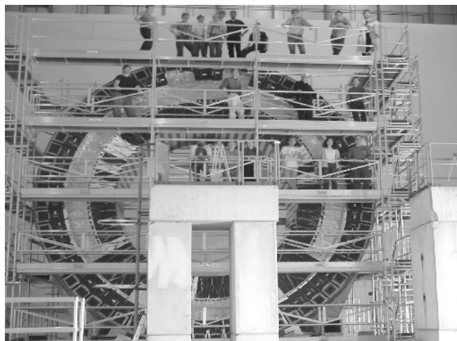
Fig. 3. The first completely pre-assembled extended barrel of the Tile Calorimeter placed behind the scaffolding.
