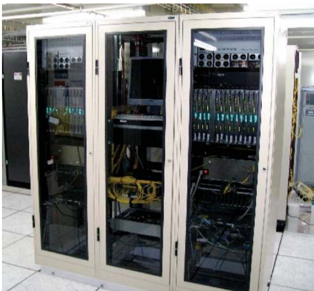
Figure 14. The CABB rack as installed in the fully shielded ATCA correlator room.
