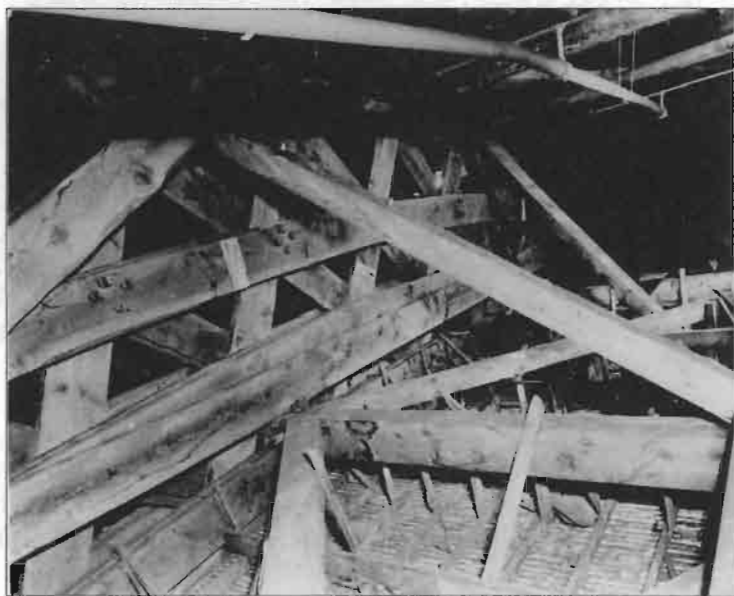
The lattice-work beams of the Tabernacle roof in cross section. Note the wooden pegs in the beams and the rawhide strips around the upper plank over a crack. Photographer unknown. Courtesy LDS Church Archives.
