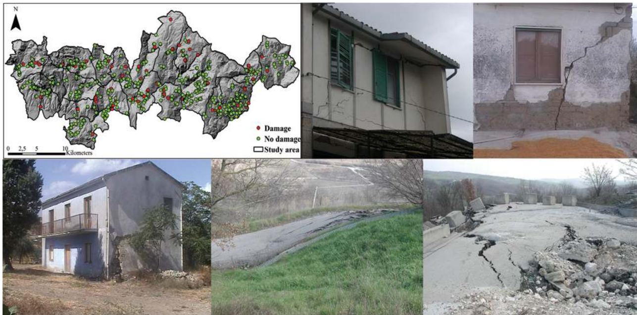
Fig. 5. Distribution of landslide-induced damages within the test area and some examples of damages recorded to buildings and roads.
