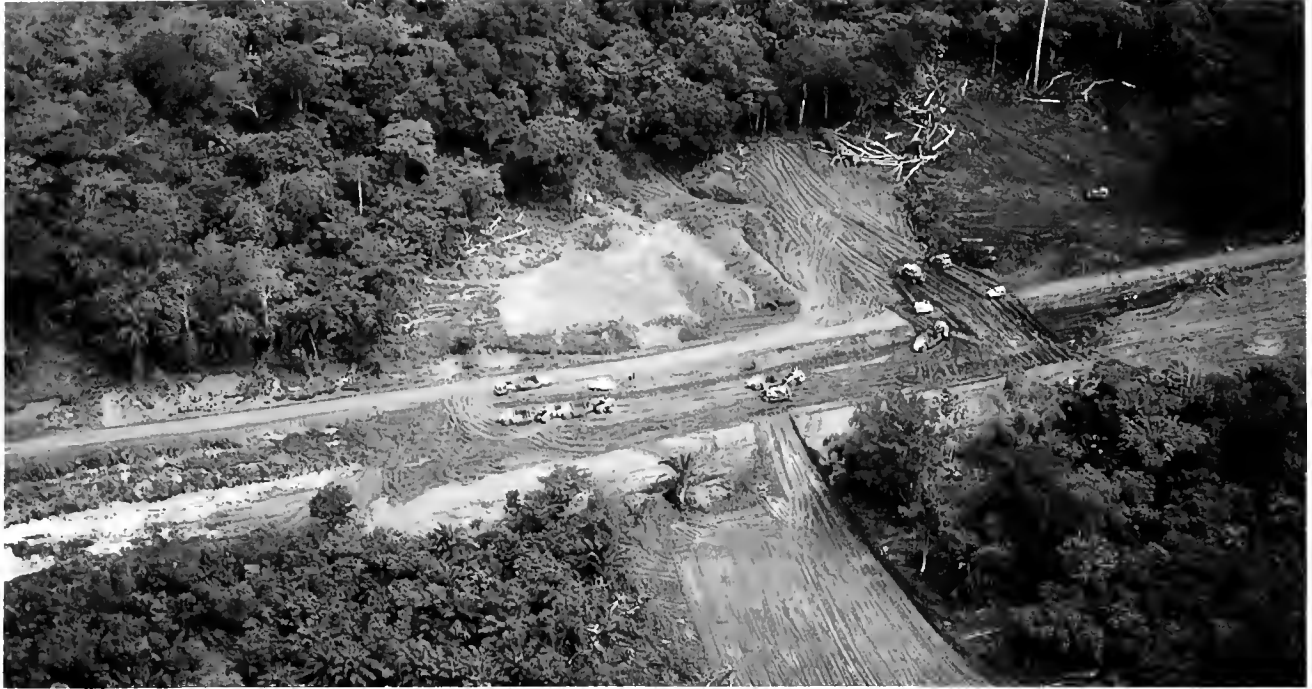
A road being built through Zaïre's rain forest. This opens the way to settlers and increased exploitation of the forest.
