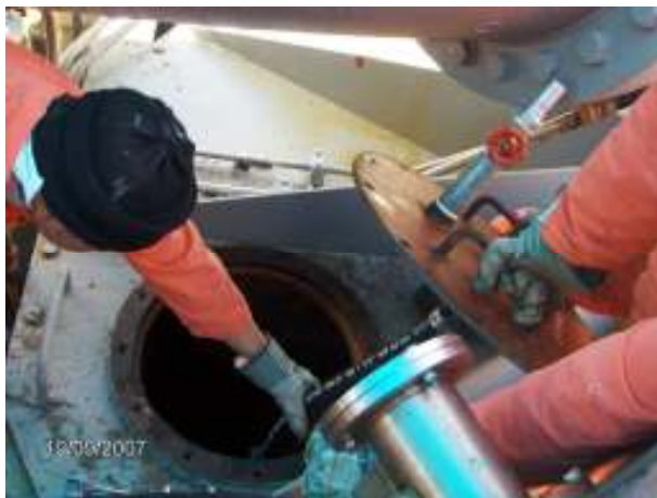
Deployment in overflow
