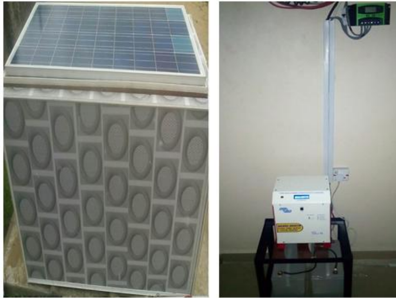
a). Solar panel on a platform 1m high.
