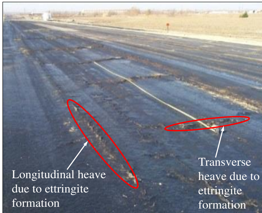
Figure 2.28: Vertical heave due to ettringite formation in sulphate bearing soil treated with cement in Texas, USA (After Harris et al. 2006)
