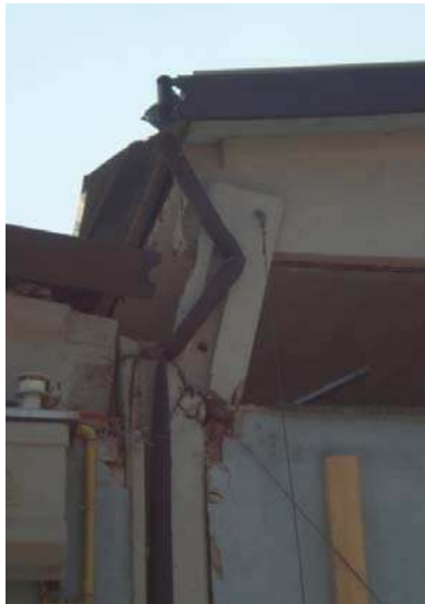
Figure 9. Shear collapse of column due to the interaction with infill masonry panel.
