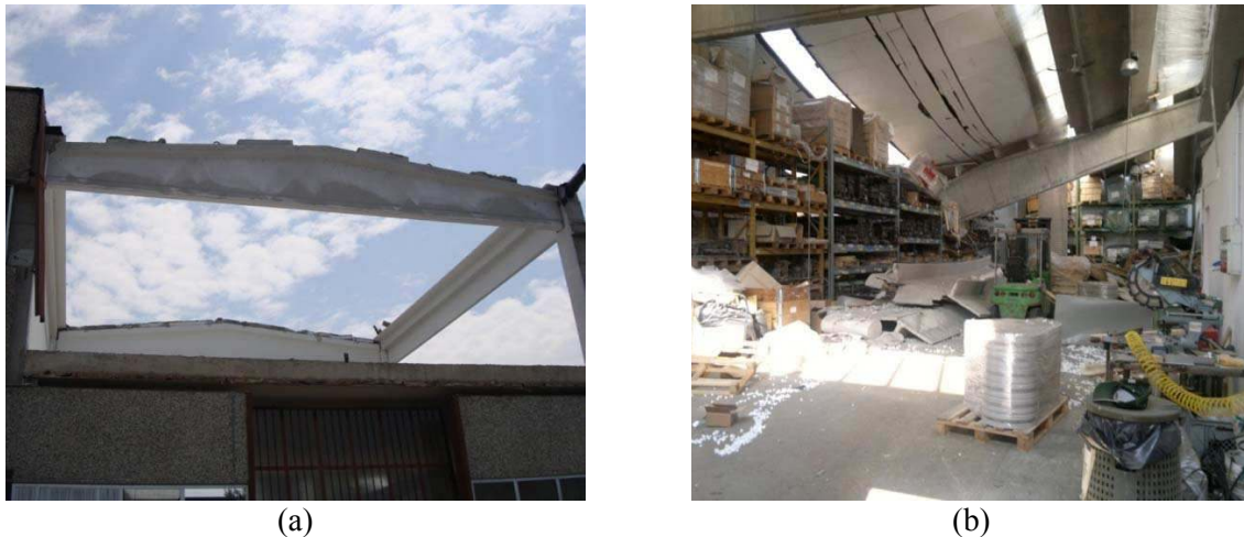
Figure 5. (a) Roof elements collapse due to the loss of support from main beam. (b) Loss of support of beam from column.
