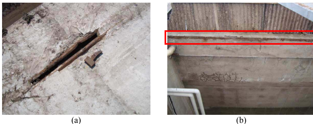
Figure 12. Collapse of vertical precast panel connection: (a) the anchor channel embedded in the panel and the failed hammer head element; (b) profile located in the beam which the hammer head elements are welded to.
