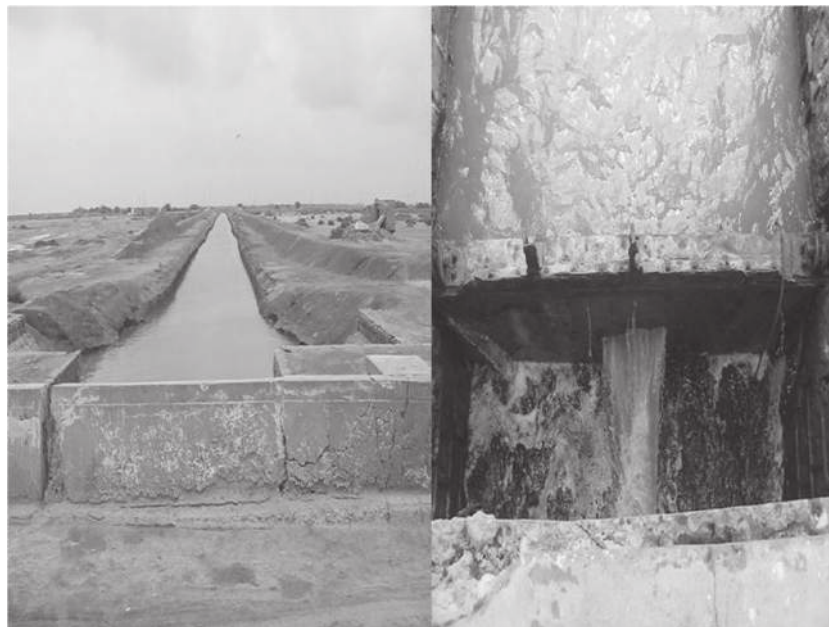
Figure 16.5 One of the drainage canals in the Indus deltaic area of Keti Bandar where the sea water is entering irrigated land through a defective gate
