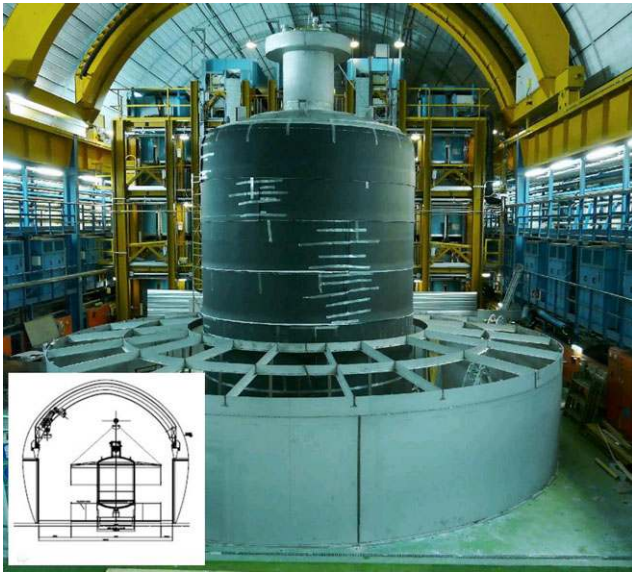
Fig. 7 The water tank under construction in Hall A of LNGs in front of the LVD detector. The inset shows how the tank is assembled from top to bottom. The hall crane lifts the upper part to which another cylinder segment of about 2 m height is welded. The cryostat in the center is protected by a black foamed plastic during the construction of the water tank
