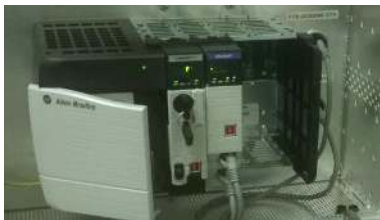
Figure 3: Allen-Bradley ControlLogix controller
