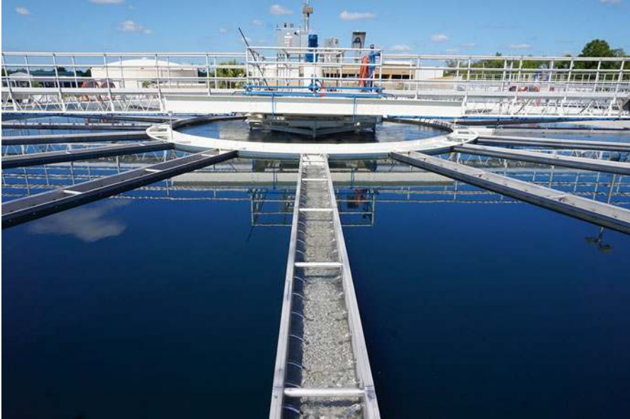
Fig. 2.2 Peace River Manasota Regional Water Supply Authority Water Treatment Plant facility. Water decontamination corresponds to one of the several regulatory costs induced by pesticide use. Estimates of regulatory costs differed considerably between studies, depending, in particular, on whether or not they considered the control of underground water. For instance, in the United States, Pimentel and coworkers began to consider the costs of monitoring underground water and wells in their papers published in 1991. The consideration of these costs led to an immediate increase in their estimates of the overall cost of pesticide regulations of more than 300 %, with these costs accounting for 90 % of total regulatory costs for pesticide use (Pimentel et al. 1991a, b). Moreover Pimentel (2005, 2009) and Pimentel and Burgess (2014) estimated that the current monitoring of wells in the United States (about US$2 billion per year) would have reached US$17 billion per year if all the wells in the United States were monitored (Unmodified photography by Florida Water Daily, under Creative Common License CC BY ( https://creativecommons.org/licenses/by/2.0/ ))
