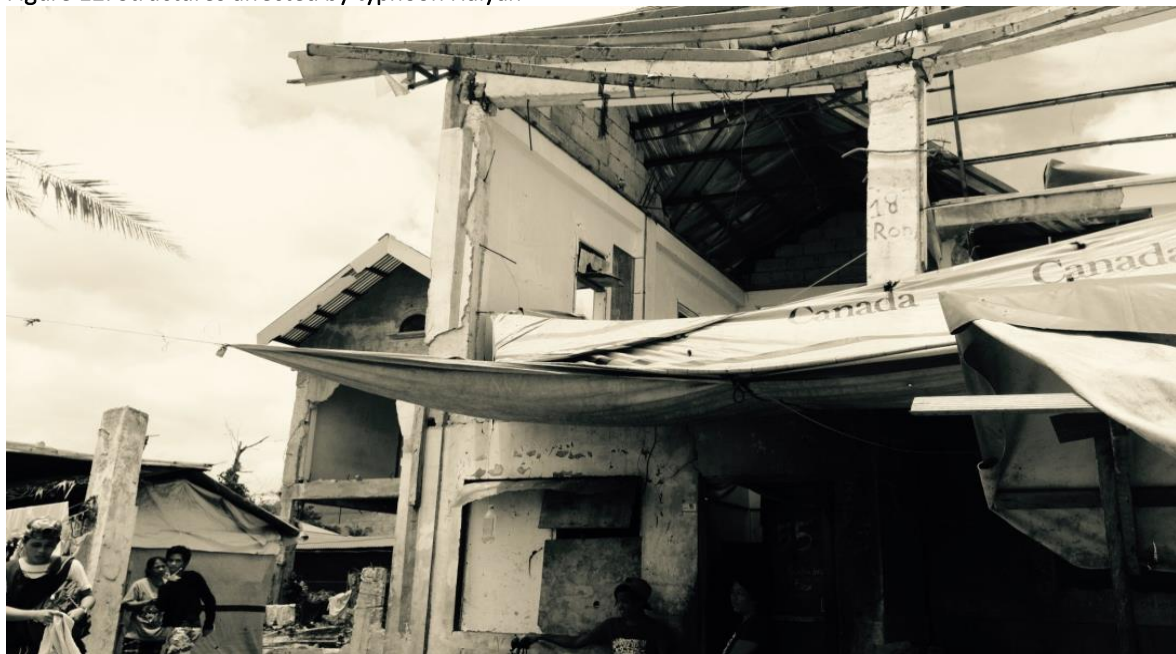
Figure 12. Structures affected by typhoon Haiyan
