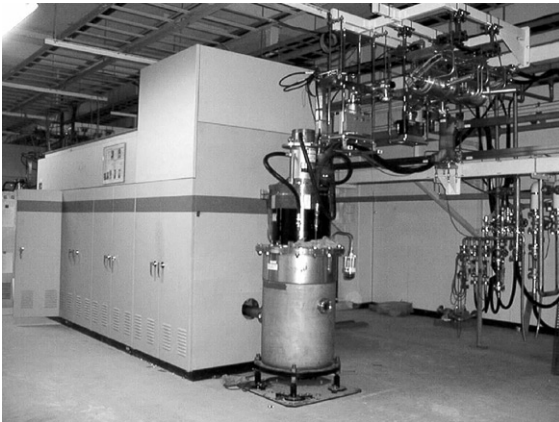
Fig. 10. The entire picture of the modulator, the klystron assembly and the SLED cavity.
