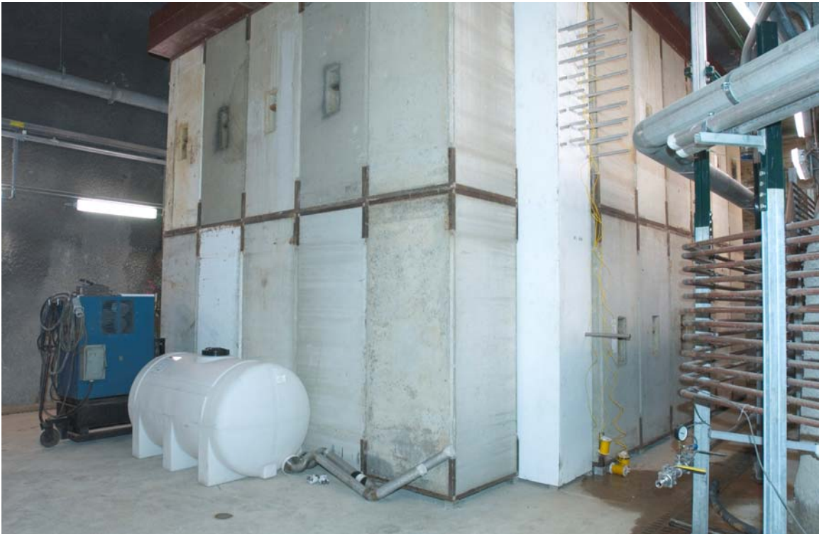
Fig 8.55: Hadron Absorber Installed
