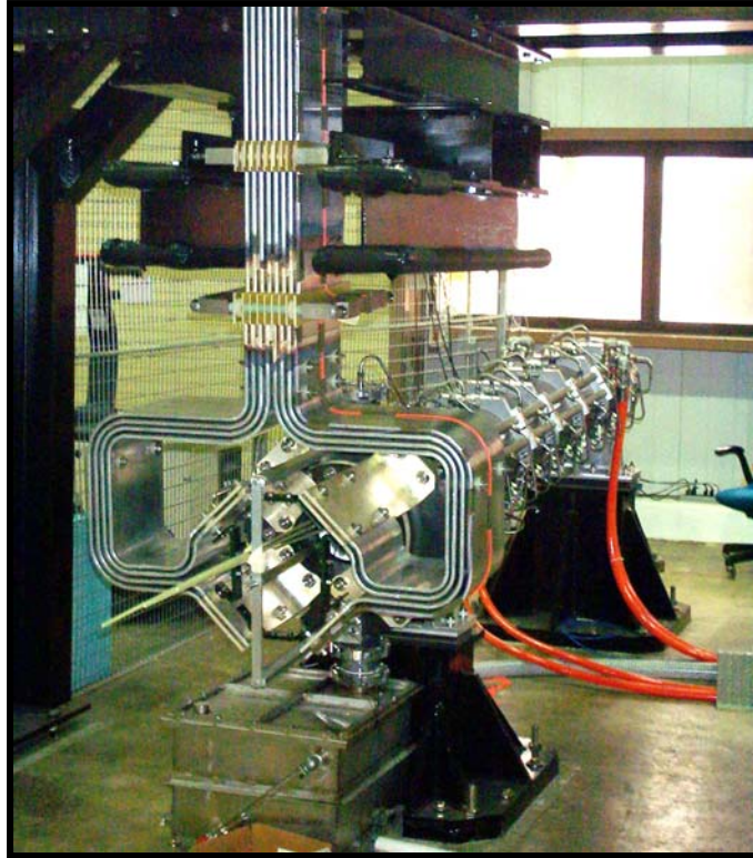
Fig 8.46: Horn 1 connected to transmission line in the MI8 service building.
