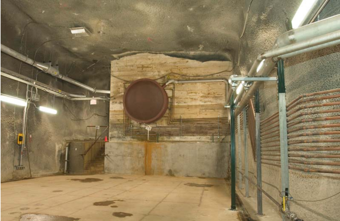
Fig 8.54: Decay Pipe Downstream Window (with decay pipe cooling pipes shown) and Absorber Hall (Hadron Absorber not installed) – emergency egress passageway on left.
