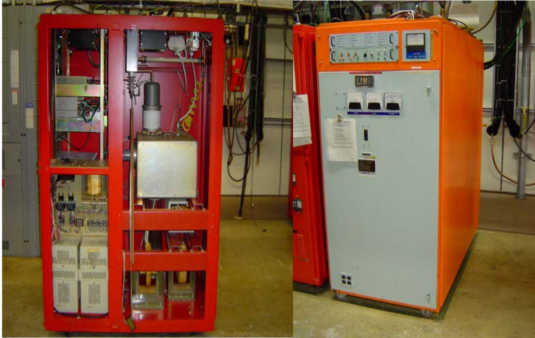
Fig 8.19: Pictures of the series tube modulator supply (left) and the bias supply (right).
