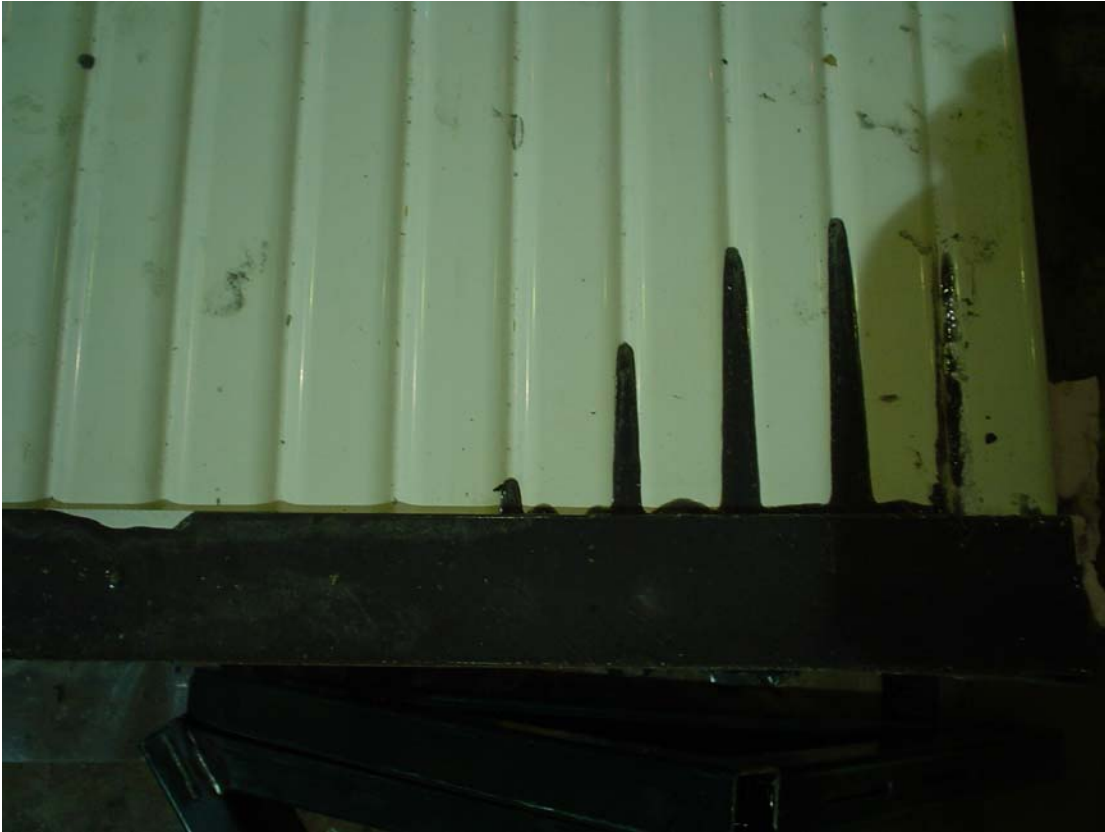
Fig. 17.114: Edge view of grout showing overfill of dam and leakage into the extrusion scallops.
