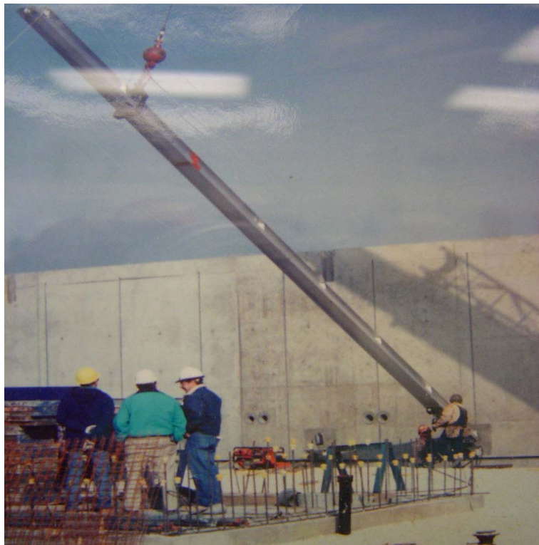
Fig 8.22: Pictures of the original bus bar installation during the construction of the MI-60 building. In the top picture the whole bus bar can be seen hanging from the crane with a support, while in the bottom picture we can see the bus bar inside its fixture for installation.
