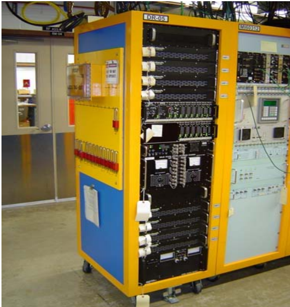
Fig 8.21: Pictures of a rack housing the solid state driver for an MI rf station.
