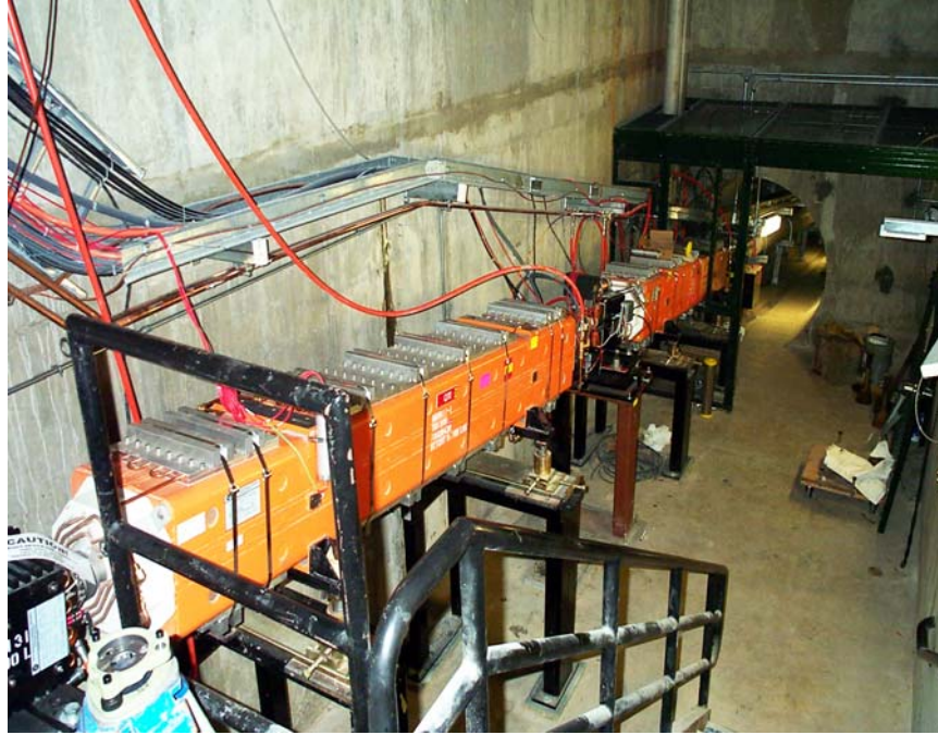
Fig 8.28: NuMI 3Q120 with External Cooling Plates
