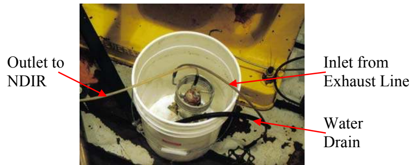
Figure 2.25. The water trap for the NDIR.
