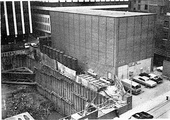
FIG. 3. View of tied-back sheet pile wall and adjacent building when excavation was almost complete.
