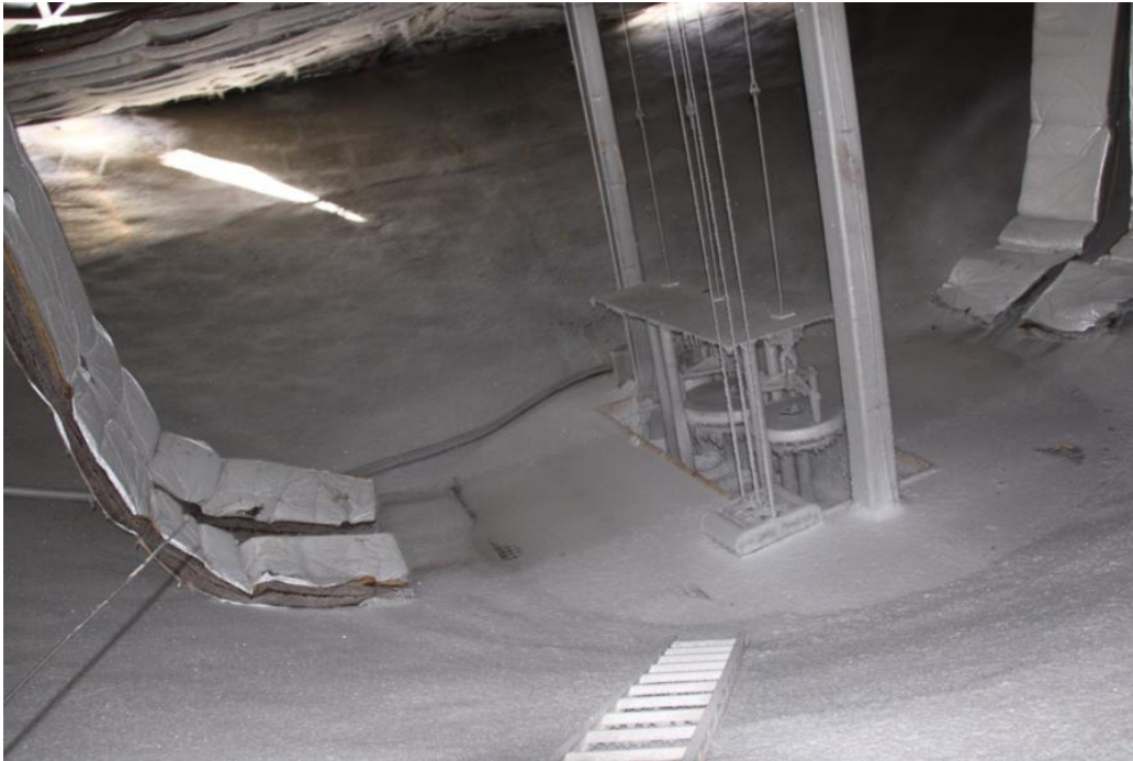
Figure 264 Inside reservoir showing dropped ceiling panels after LNG Test 2.
