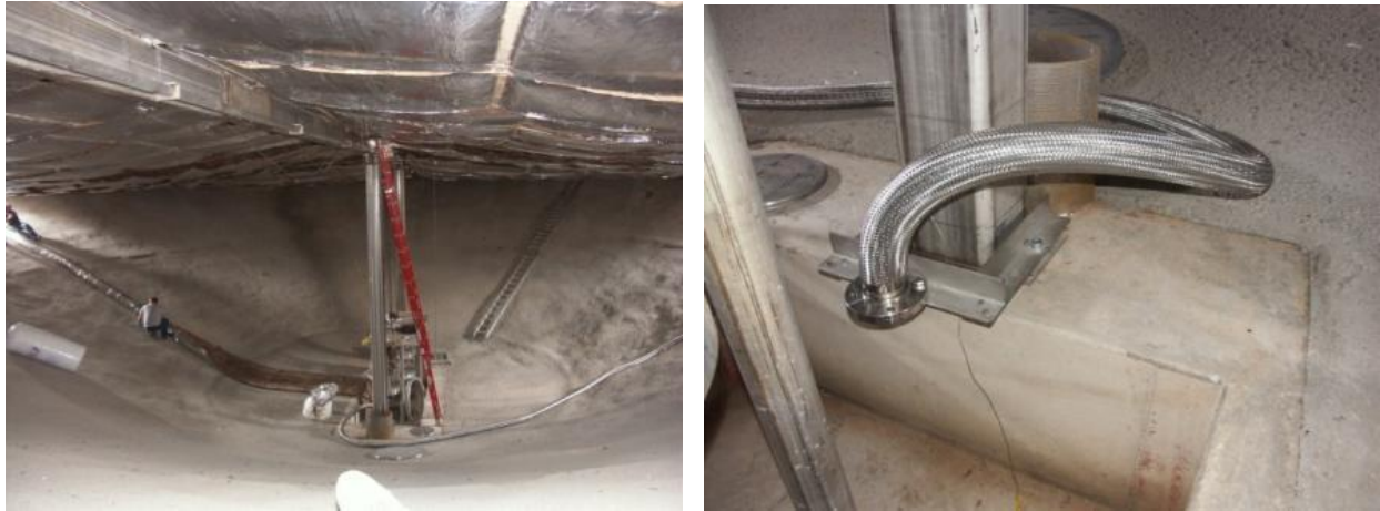
Figure 159 Hose extending to floor and discharging into well.
