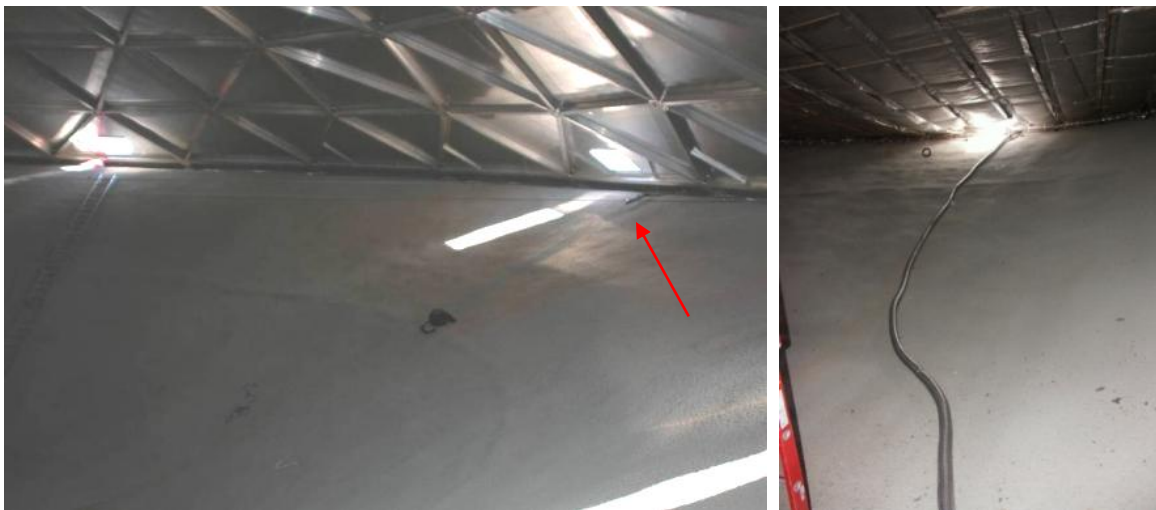
Figure 158 Original LNG discharge point and flexible hose extension.
