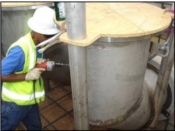
36 inch SS elbow mated to 36 inch RCP
