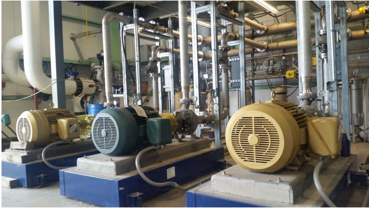
Figure 4.6: Typical LCW pump room.
