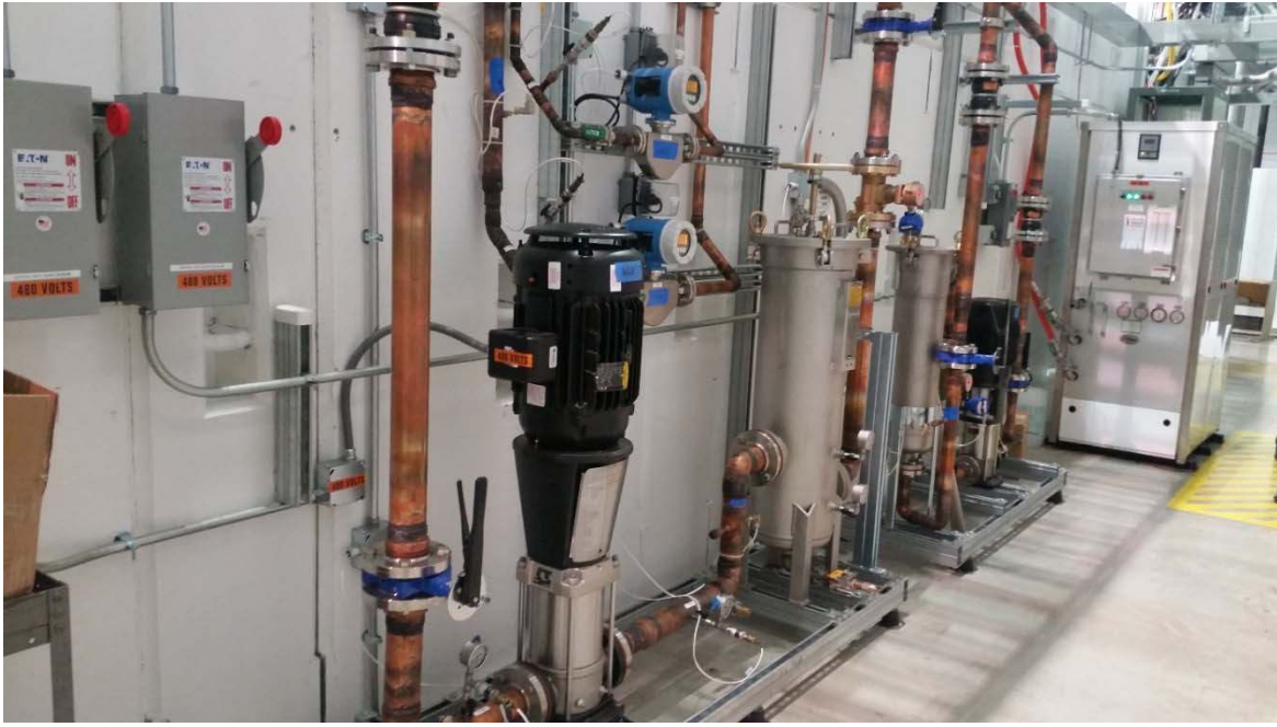
Figure 4.7: RFQ LCW showing separate Vane and Wall LCW skids. These skids incorporate pumps, filtration, and precision flow measurement.
