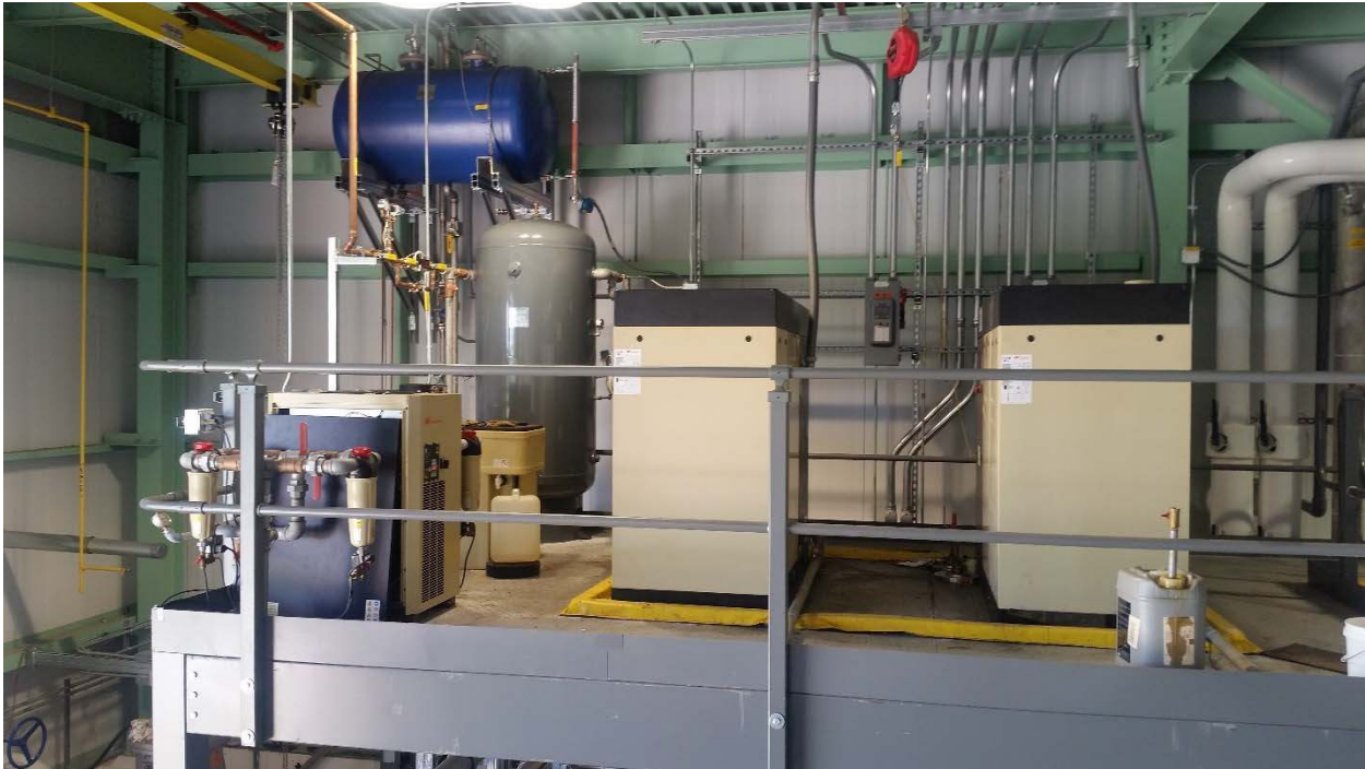
Figure 4.9: Typical compressed air arrangement. Screw compressors, dryers, filters, and distribution piping shown
