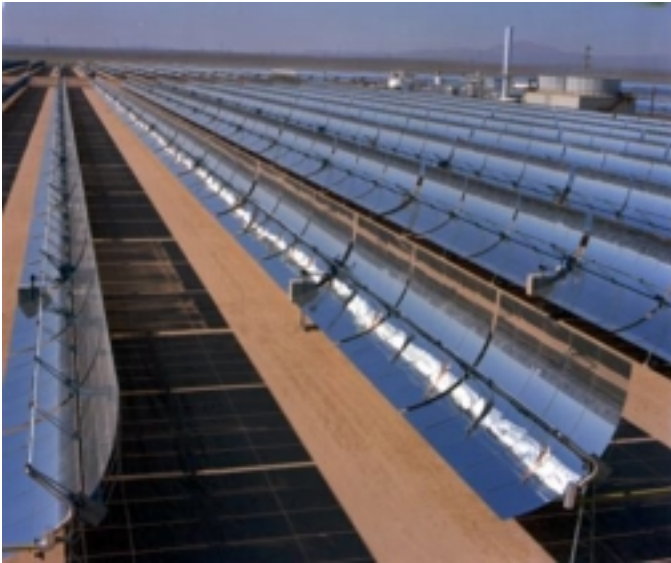
Figure 1 SEGS V Parabolic Trough Solar Thermal Power Plant [KJC Operating Company]
