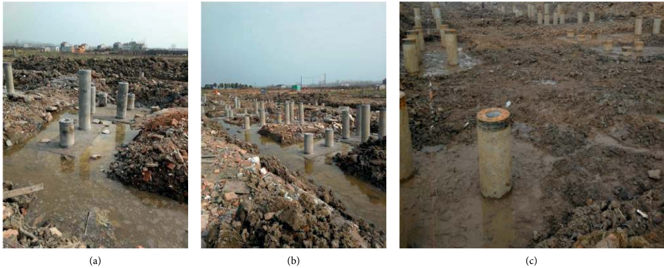
FIGURE 1: The buried depth of piles in the site varied greatly.
