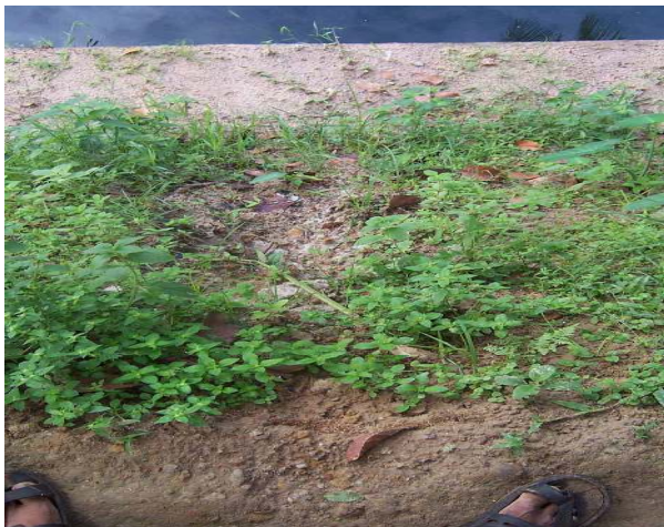
Fig. 11. CP- less density, non uniform vegetation with soil erosion, after 7 months.
