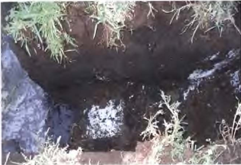
Plate 5.5: Trench showing section of lime-fly ash barrier at 1m below ground surface. Grout at upper right hand corner from an adjacent injection hole.
