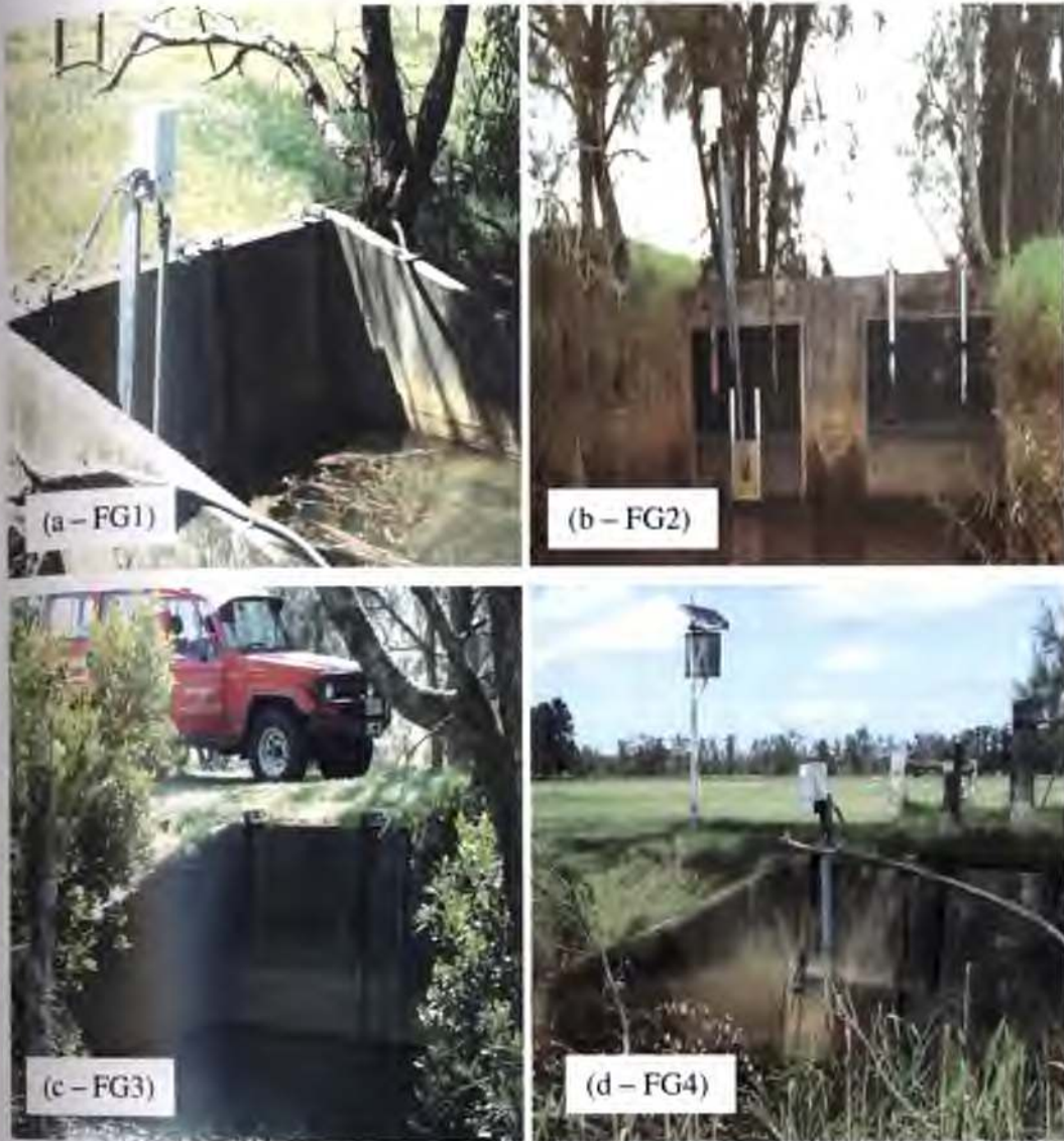
Plate 4.4: Tidal restricting floodgate installed on flood mitigation drain in the Broughton Creek Estuary. Floodgate (a - FG1), modified floodgate is located downstream from the Lime Injection Site. Floodgates (b - FG2), (c - FG3) and (d - FG4) are the other floodgates monitored during this study
