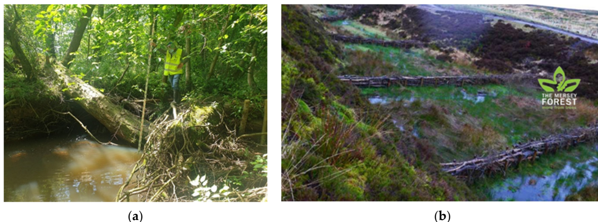
Figure 2. Large woody/engineered log barriers: (a) Tees Rivers Trust in Coatham Beck, Co. Durham, in collaboration with EA, Forestry Commission, Stockton Borough Council, Arup and Newcastle University; (b) Smithhills, Mersey Forest, Liverpool University and EA [46] (photo by Norbury).
