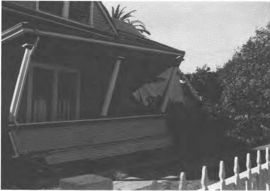
FIG. 6. Collapsed cripple wall and porch in a residence at Main Street in Los Gatos.
