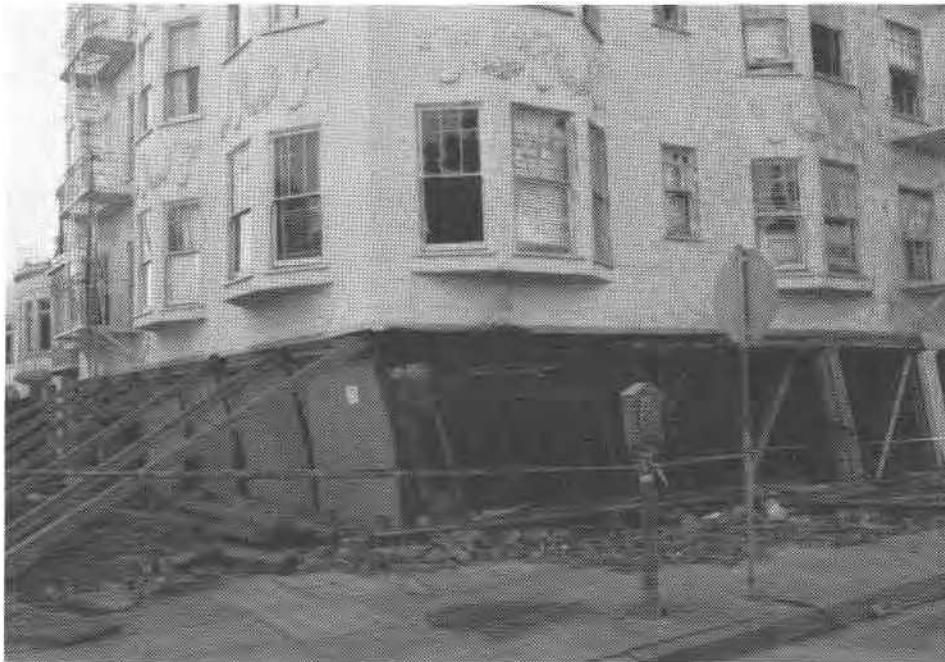
FIG. 7. Near collapse of a four-storey wood frame apartment building at the corner of Beach and Broderick streets, Marina District, San Francisco.
