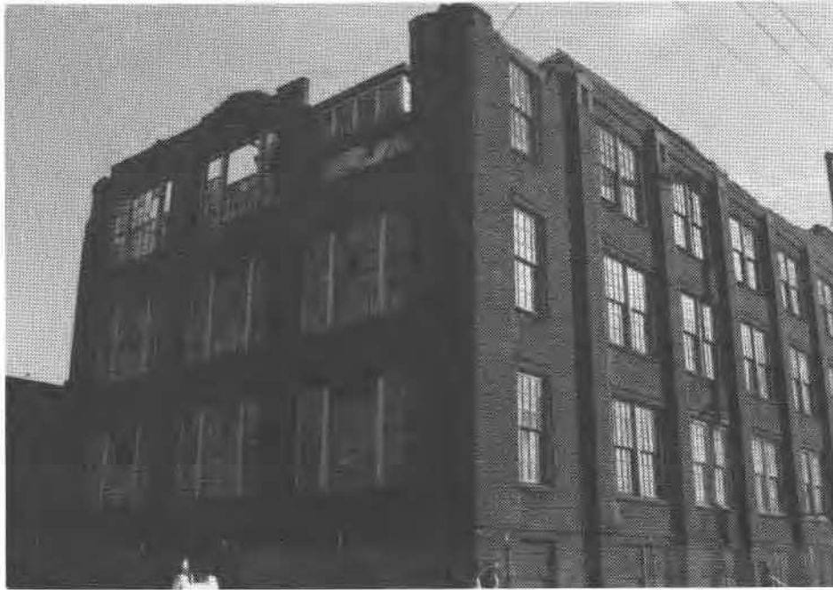
FIG. 8. Collapsed roof caused damage to the lower floors in the unreinforced masonry building on Campbell Street in Oakland.
