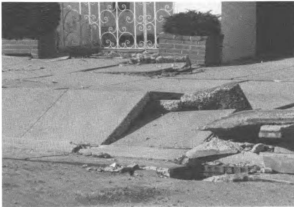
FIG. 5. Buckled pavement, Marina District, San Francisco.
