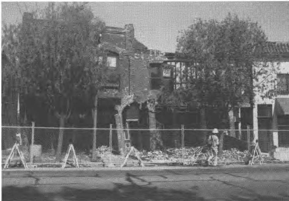
FIG. 9. Major damage to unreinforced masonry wall building, 39 Main Street, Los Gatos.
